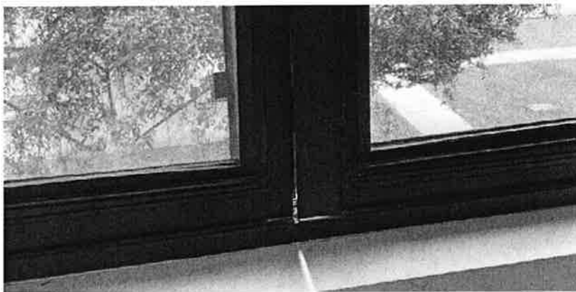
Window frame separation
